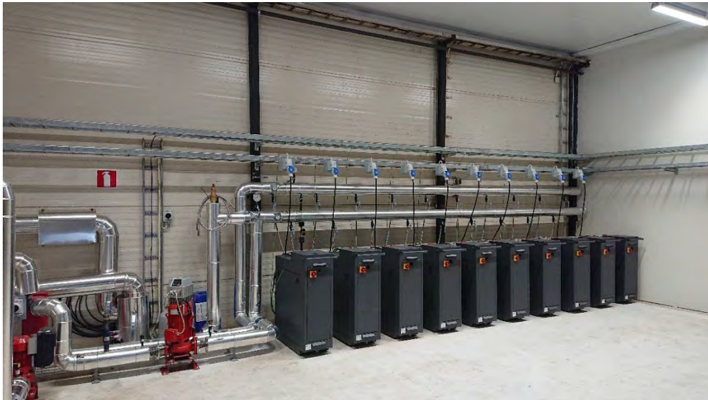
Figure 8. Kuulea Distributed Data Centers with Heat Recovery. Image: Kuulea.
